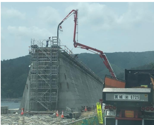
Figure 3 Construction of a coastal levee in Ishinomaki City, an example of infrastructure projects that dominate reconstruction.
